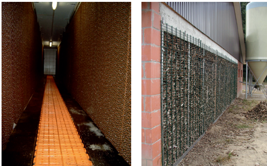
Figure 6: Three-stage facility indoor/outdoor view (photo DLG)
