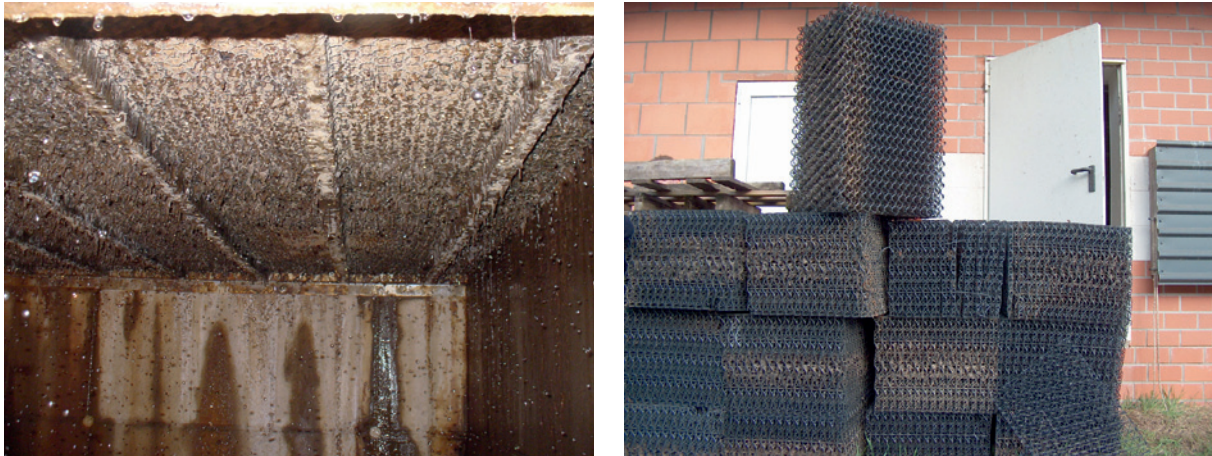
Figure 8: Partially clogged packings (photo left Dr. Hahne, photo right DLG)
